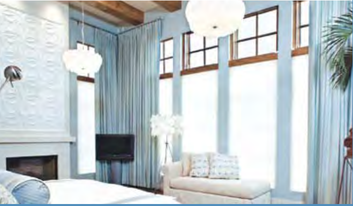
The motorized shades in this master bedroom are integrated with the home automation system.
